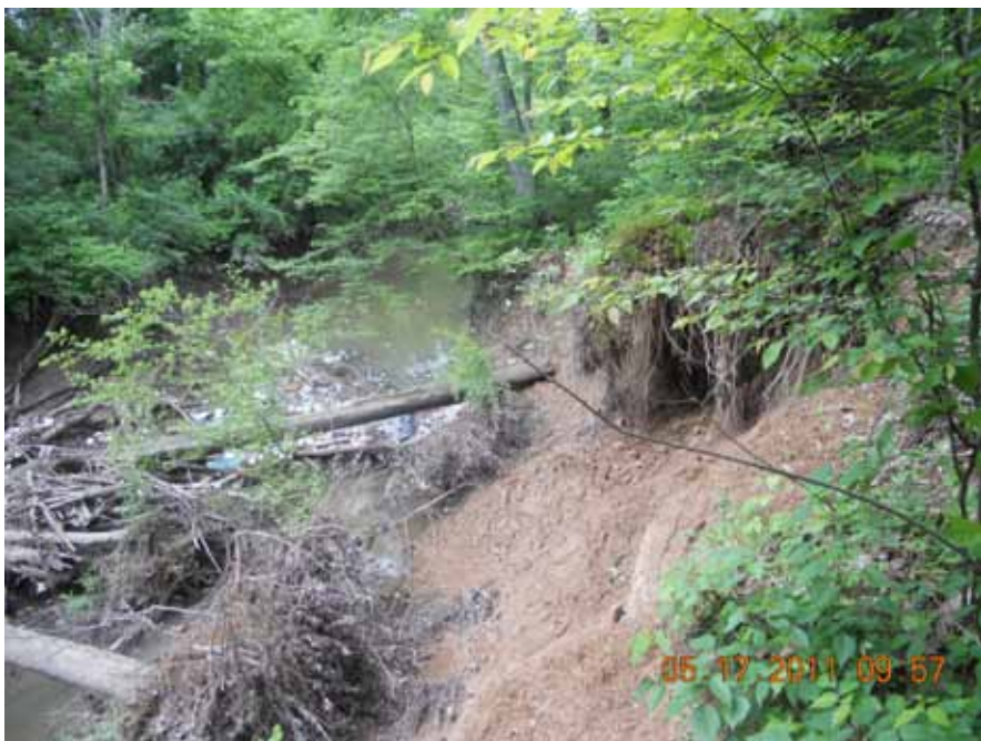
Erosion along Mill Creek
