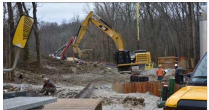
Shaft to access break along Harrods Creek
