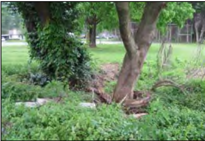
Sinkhole located near existing tennis court location
