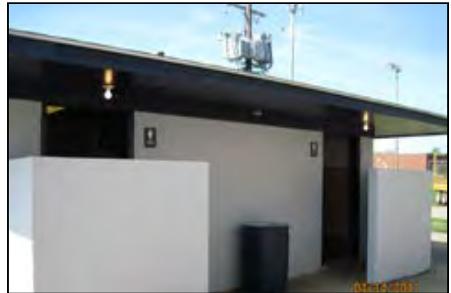
Existing restrooms at main concessions
