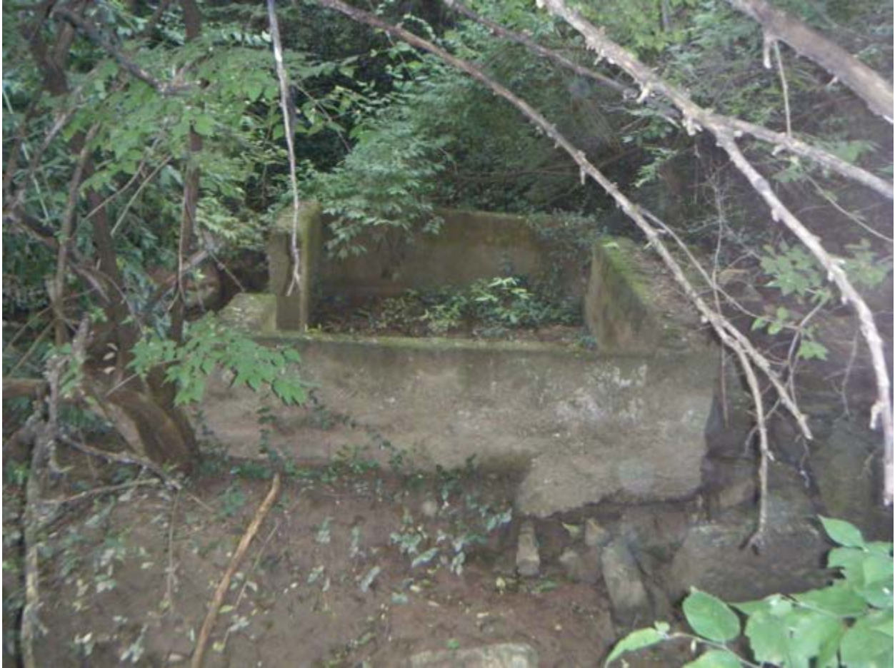
Figure 79. Foundation at base of large sinkhole, facing northeast.
