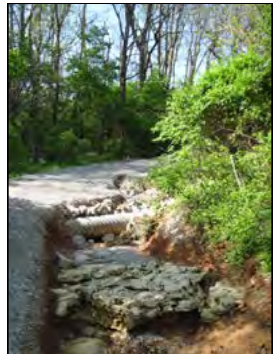
Drainage issues along access road to practice fields
