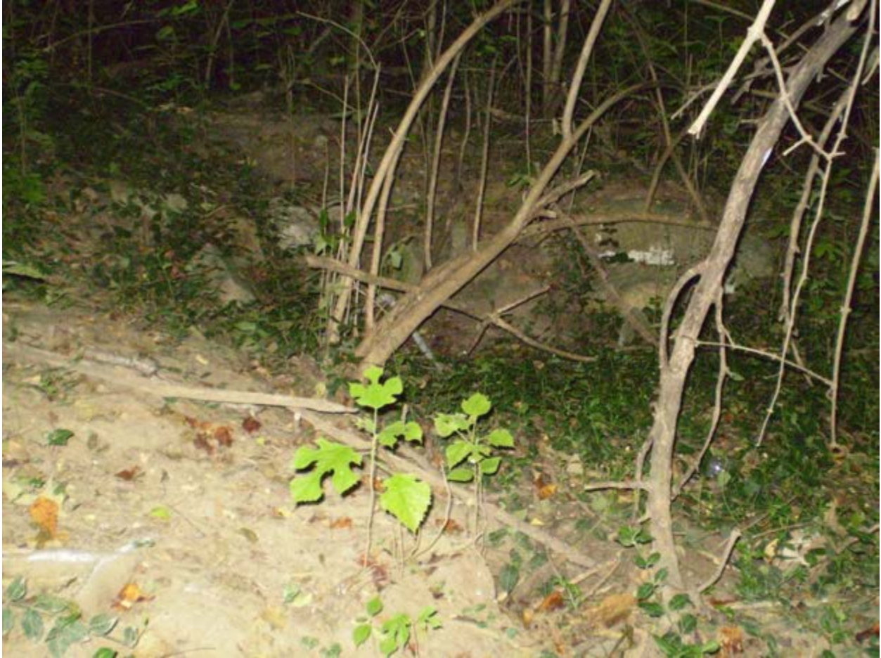
Figure 74. Northeast corner of house foundation and depression.
